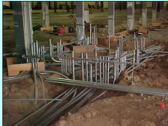
Early meticulous planning allowed conduits to be run before concrete was poured.
